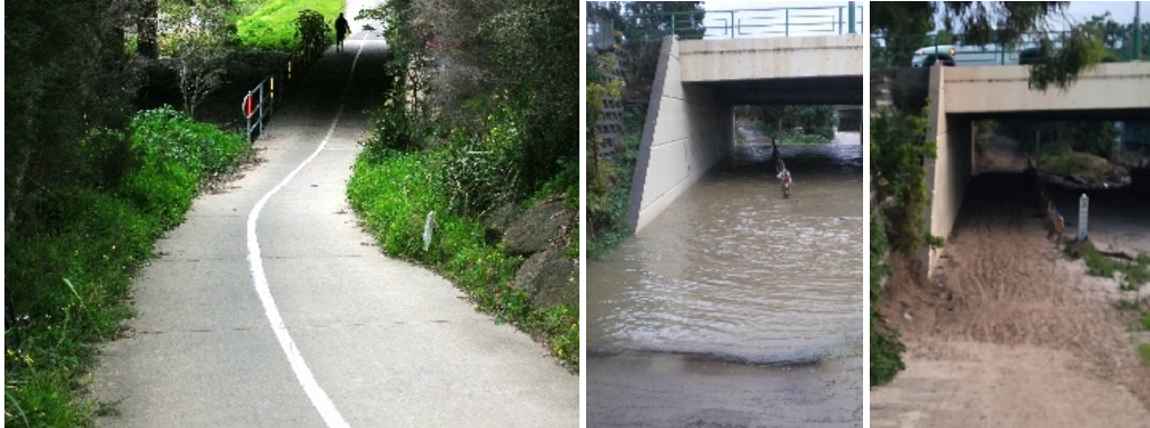
Figure 4.1 – Gardiners Creek Underpass Concerns
