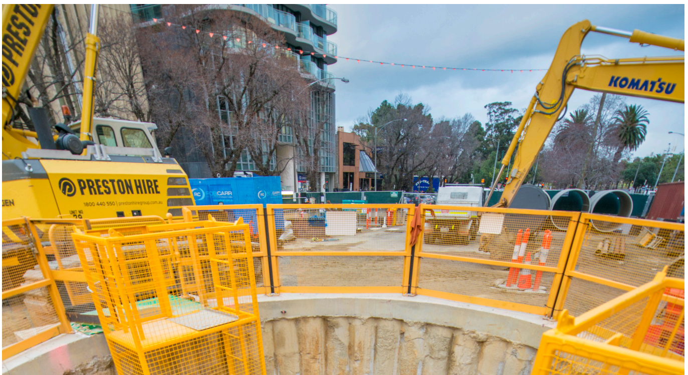
The South Yarra Main Sewer being relocated for the Metro Tunnel Project.
