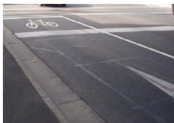
Loop detectors in the road at Victoria St, Richmond
